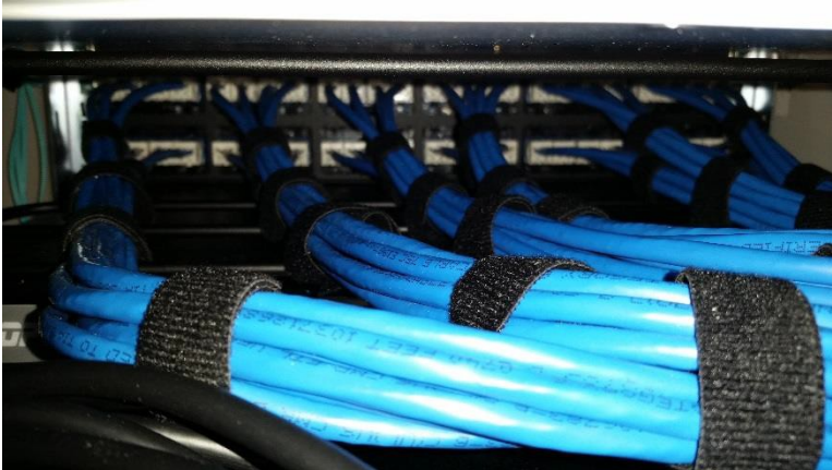
Figure 15: Copper Cables Tak-Ty to the Strain Relief Bars
