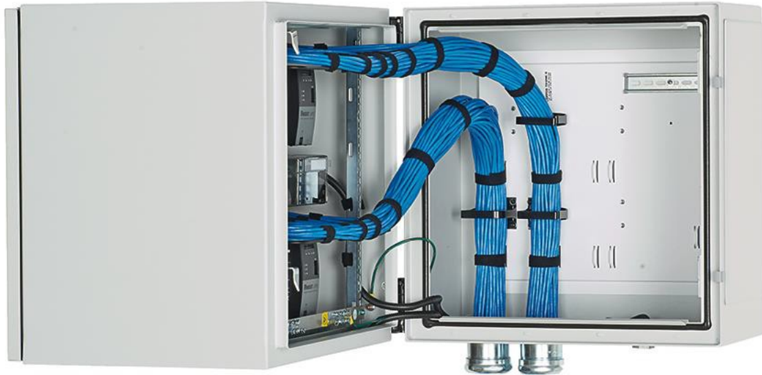
Figure 14: Copper Cable Routing showing Copper-A on the left and Copper-B cables on the right.
