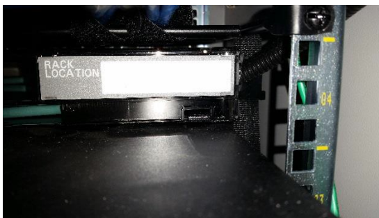
Figure 7: Loom tubing routed around hinge point and rail.
