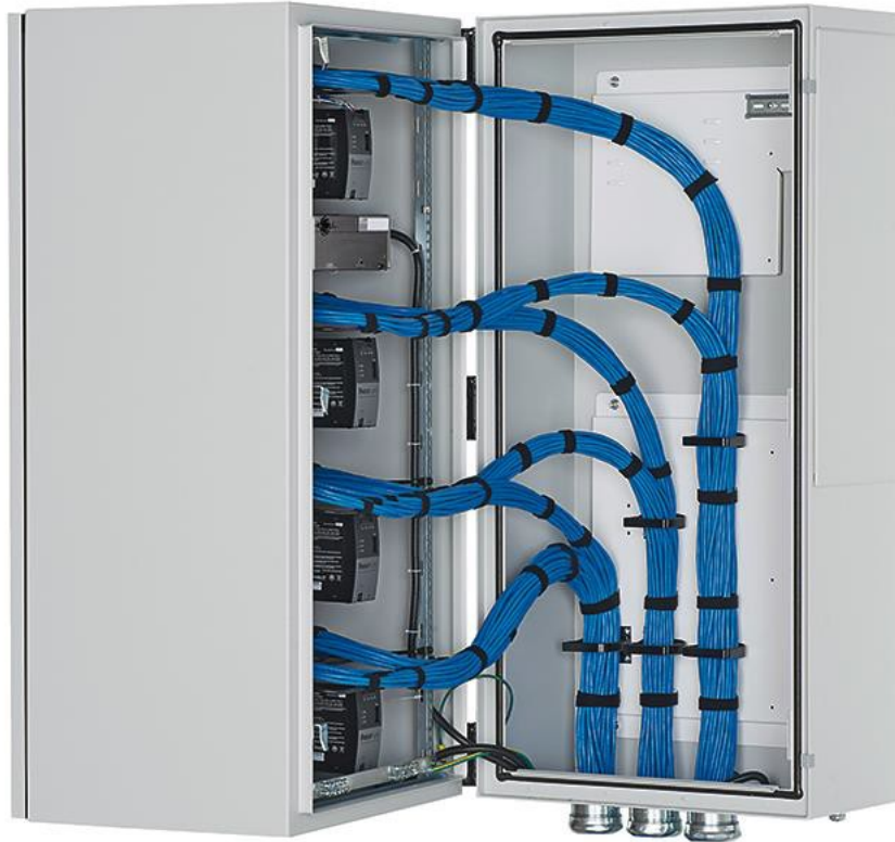
Figure 14: Copper Cable Routing showing Copper-A on the left and Copper-B cables in the middle, and Copper-C cables on the right
