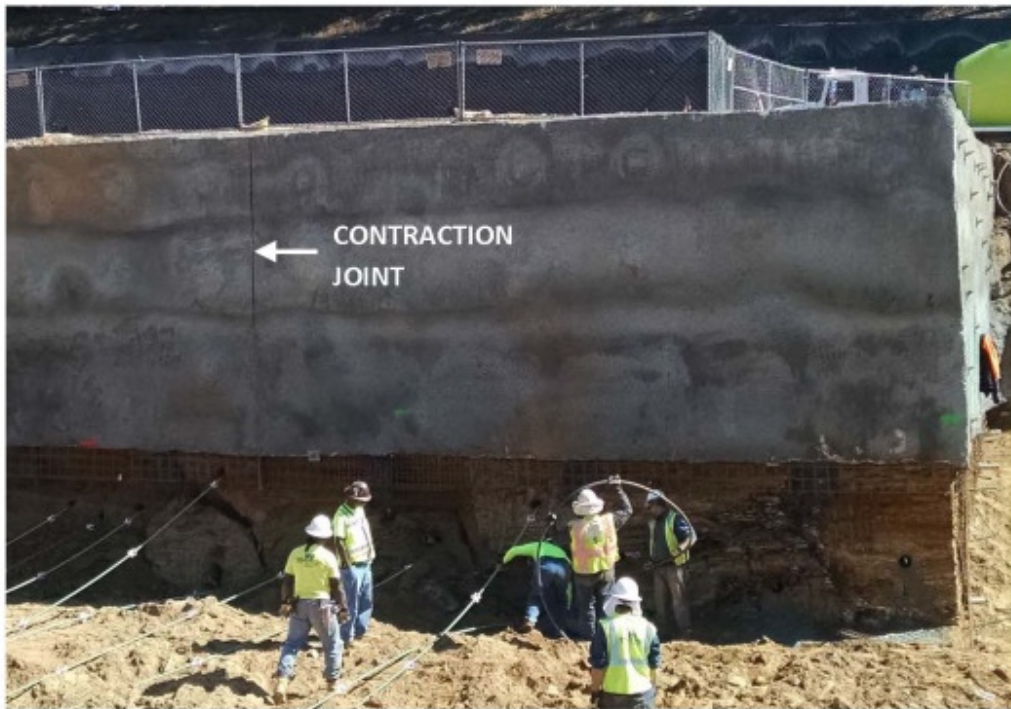
Photo 2 – Contraction Joint in Right-Angle Soil Nail Wall
