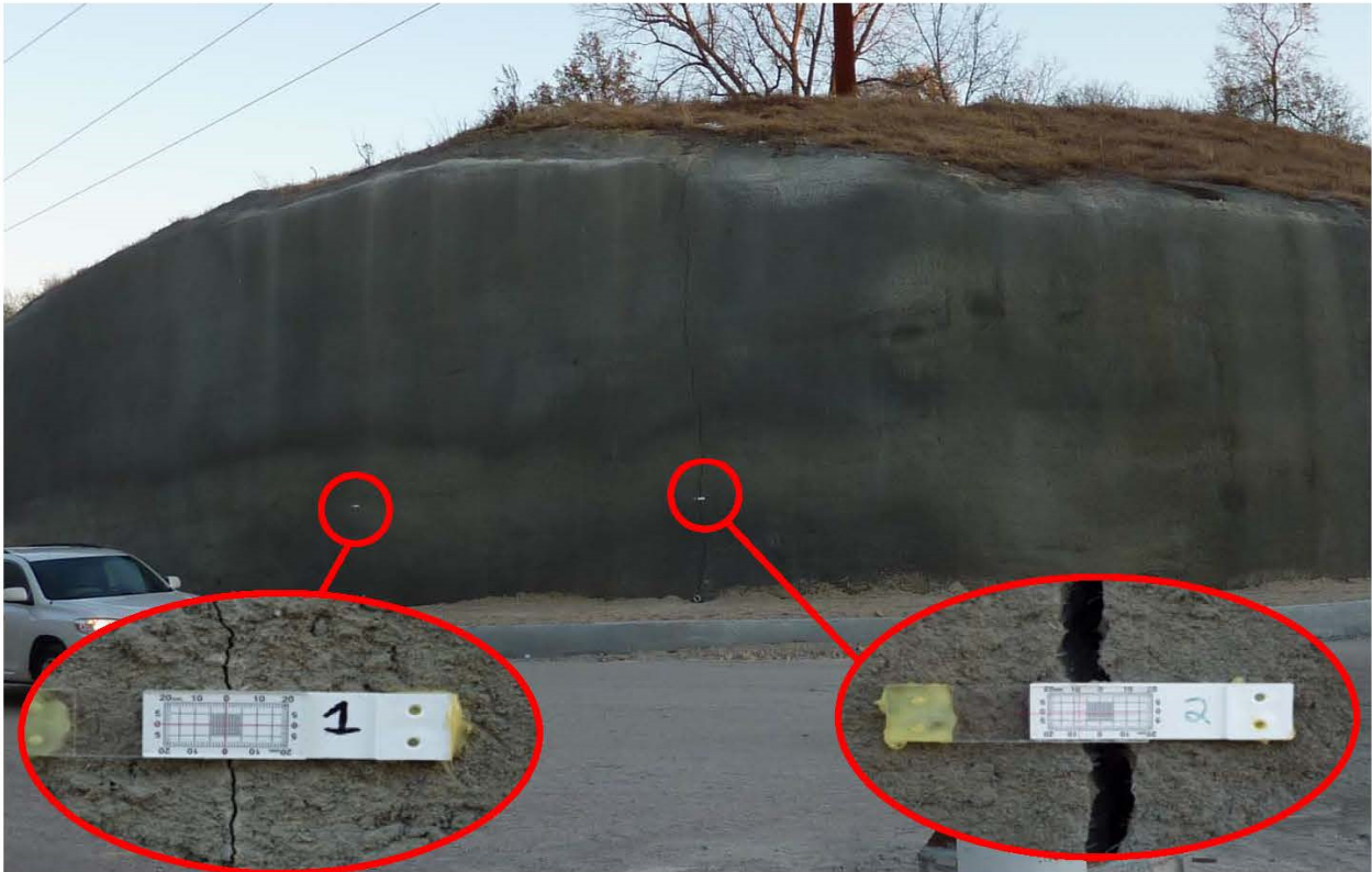
Photo 7 – Curved Wall with Unanticipated Joints Developing
