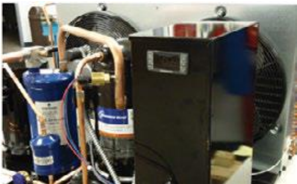
Figure 11 Large Black Electrical Box
