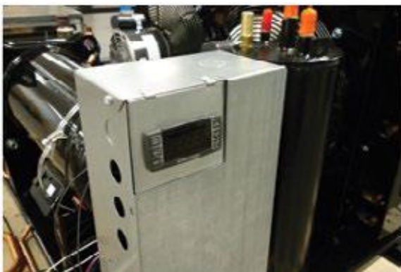
Figure 9 Silver Electrical Box
